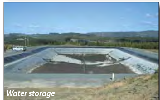
Timber treatment plant
